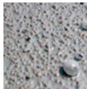
Swelling due to sand on undercoating and the gap between sand particles
