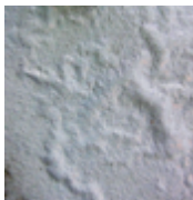
Expansion due to moisture on lower surface
